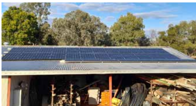
10Kw solar system at Bingara sewerage treatment plant
