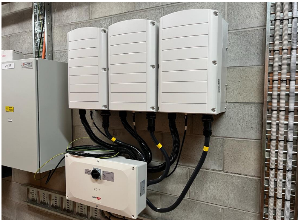
Solar system at Bingara Water Treatment Plant
