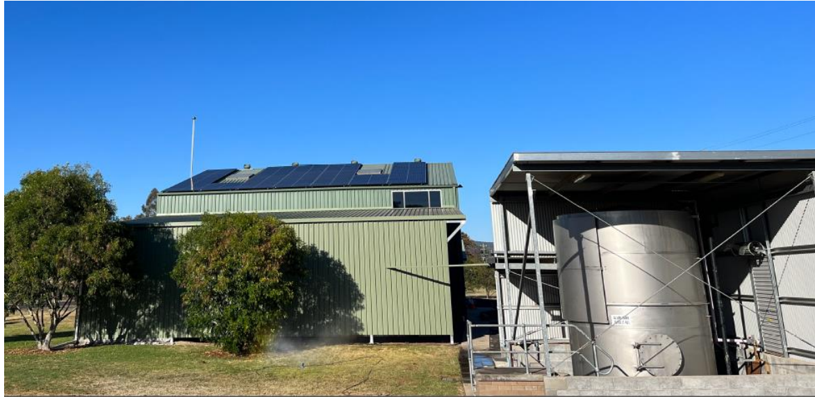
New solar panels on Bingara Water Treatment Plant
