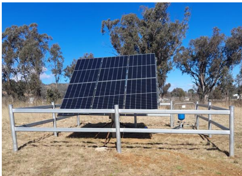
Upper Horton solar bore
