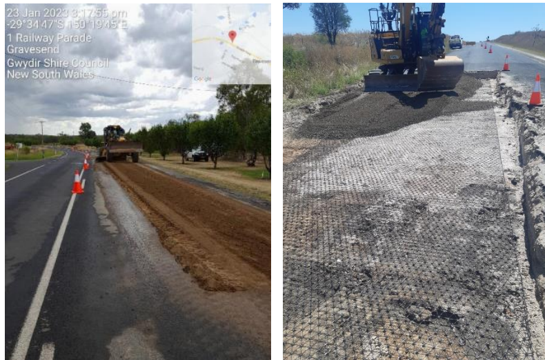
Heavy Patching, Gwydir Highway and North Star Road
