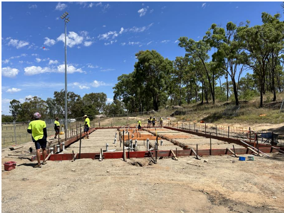
Nicholson Oval Amenities – Preparation of the footings, slab and underfloor plumbing and drainage.
