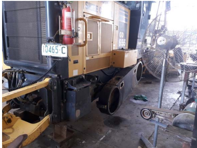
P1464 Grader - replacement of bearings seals and brake linings in the tandem drive
