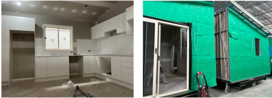
The new Bingara Caravan Park residence being built onsite at Uniplan in Armidale.
