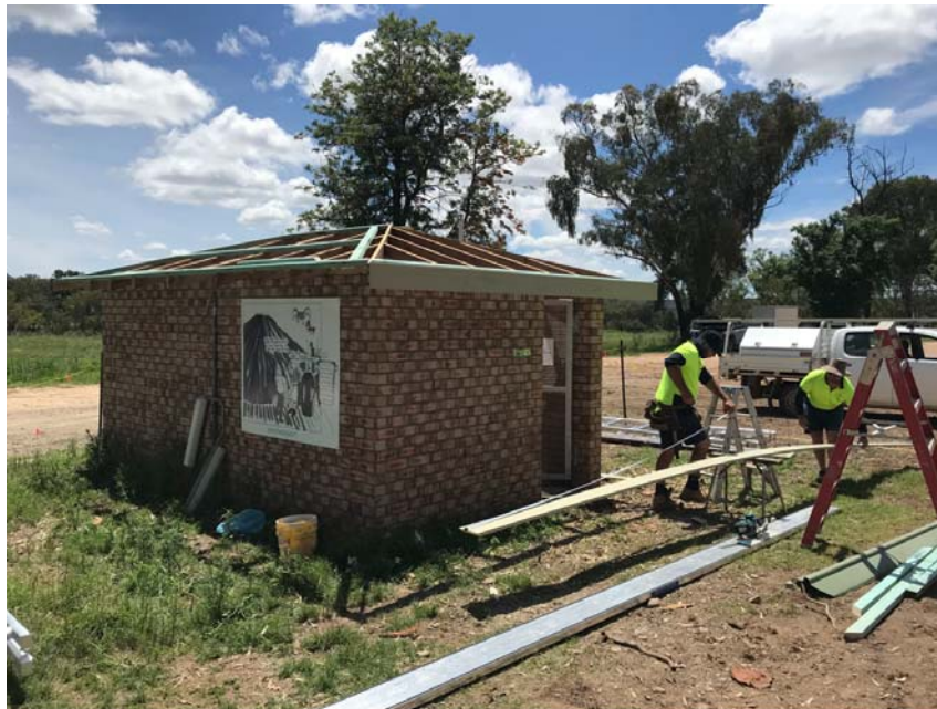
Warialda Saleyards amenities – repairs being undertaken after a tree fell on the building
