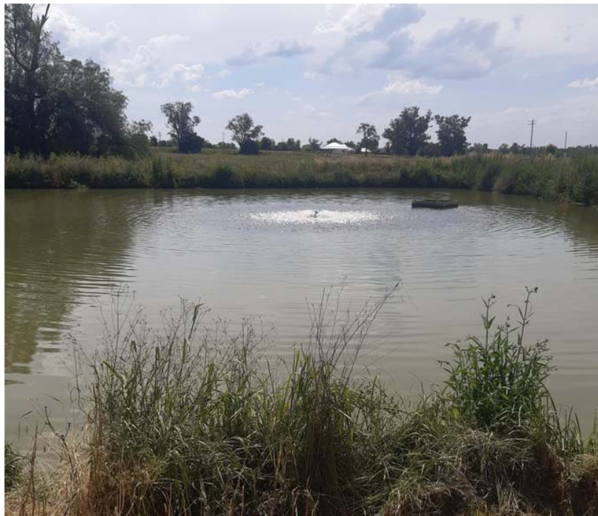
Aerator at work in Pond 2 at the Sewerage Treatment Works, Bingara
