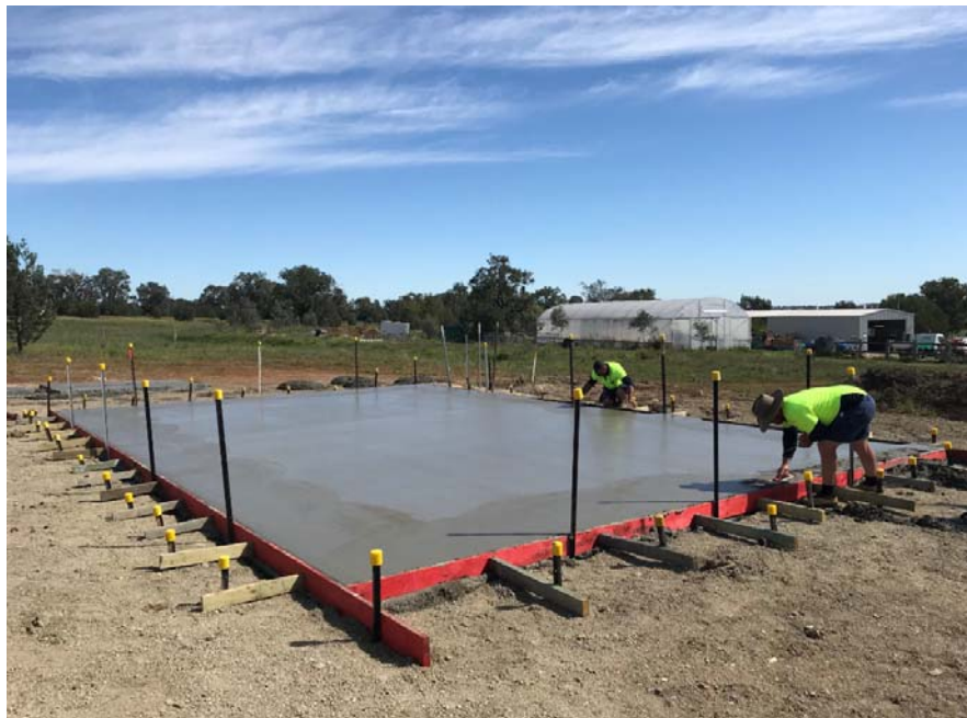
Laying of the slab for the "Meat Shed" at the Living Classroom
