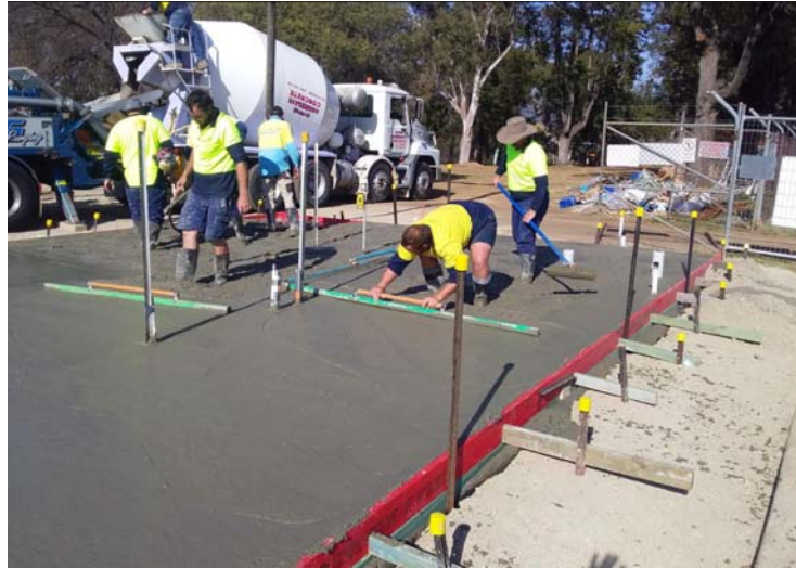
Laying of the slab for the administration building and kiosk at the Bingara Pool
