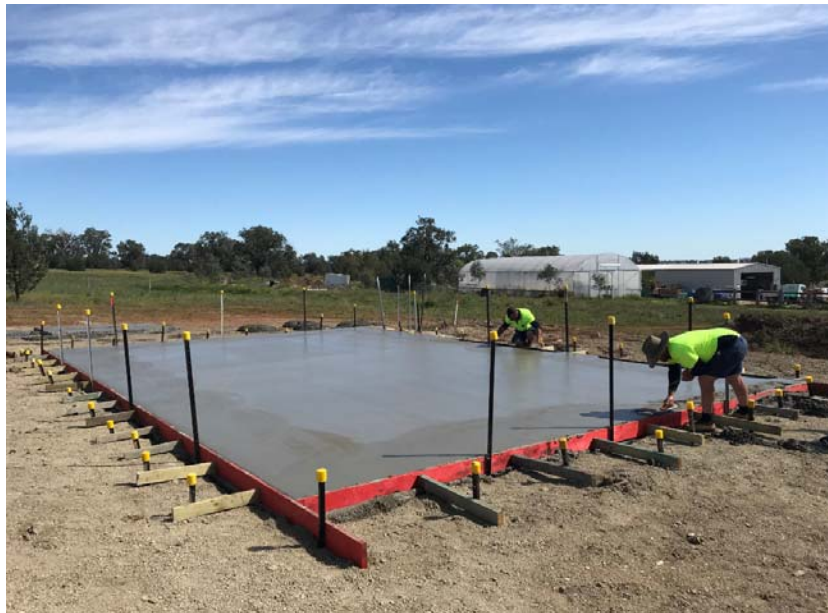
Laying of the slab for the "Meat Shed" at the Living Class
