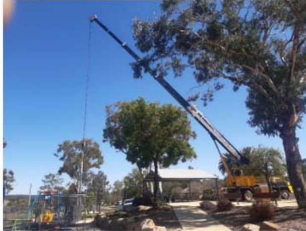
Installation of the poles for shade shelters in All Abilities Park, Warialda
