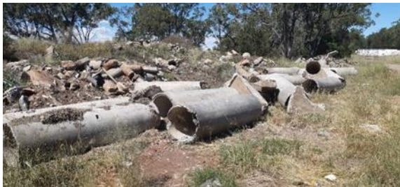
Croppa Creek: Pipes being dumped from upgrade to I B Bore Rd.
