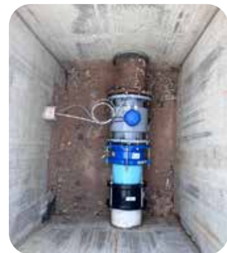
Warialda South Reservoir outlet meter
