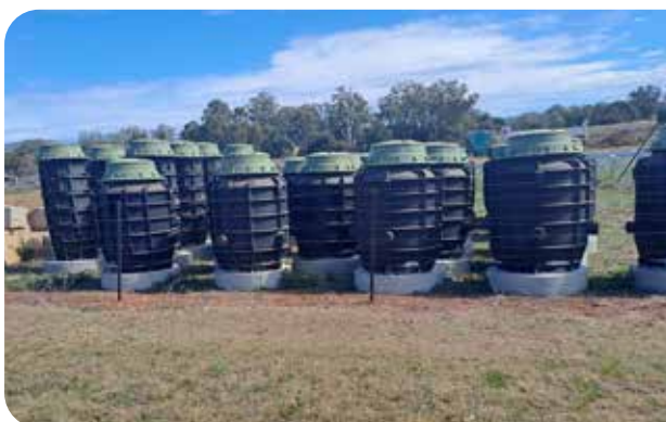
Pressure sewer pump stations
