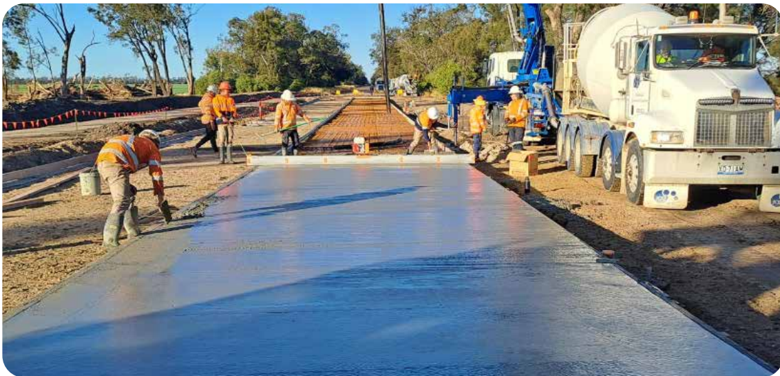
County Boundary Road Floodway 6 – placement of concrete on the western side of the new causeway.
